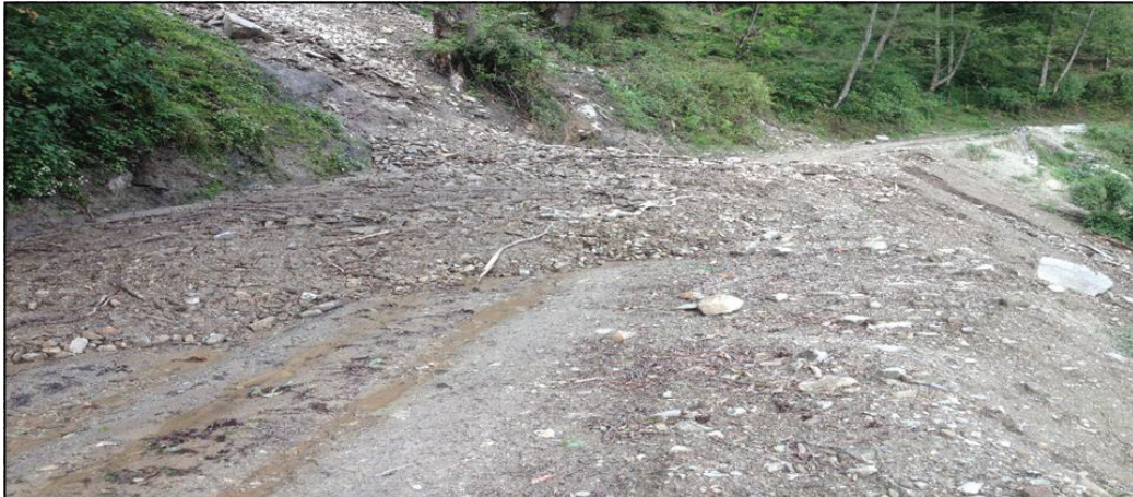
Figure 11: Landslides from road erosions
