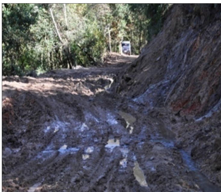
Figure 19. Poor road drainage on a farm roads
