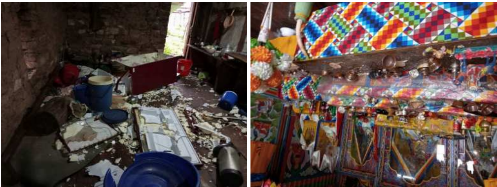
Figure 5: Damage caused by bear
